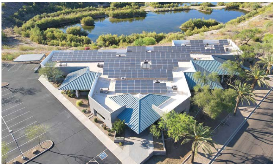
More than 8,000 square feet of solar panels, which produce 86,000-plus kilowatts annually, adorn the roof of Fruth Group’s state-of-the-art facility
